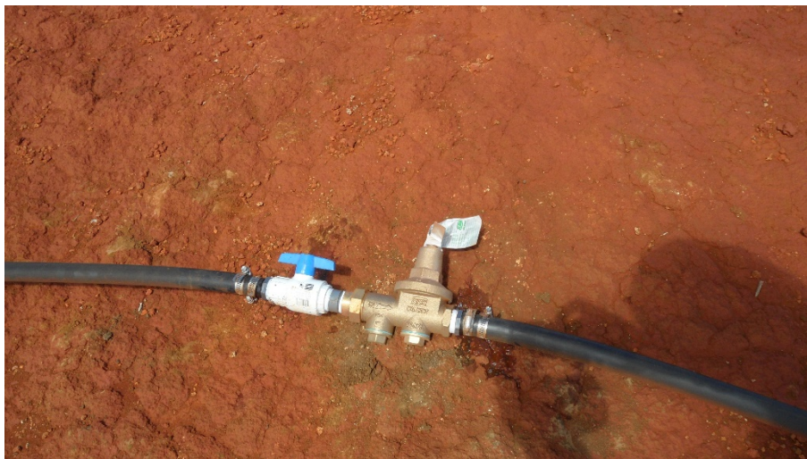
A pressure reducing valve on the 1" sub main to alleviate high pressure blow outs in the irrigation line.
