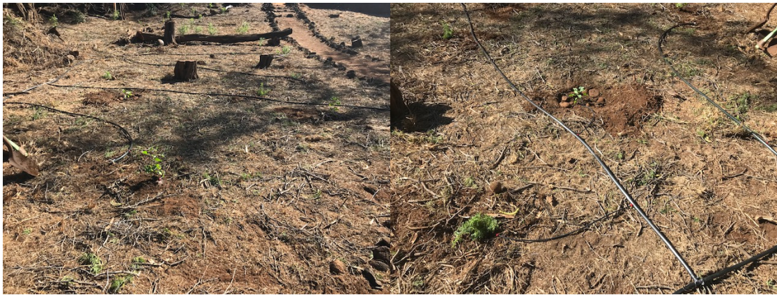
Top Left: laying irrigation line for new plantings Top Right: Completed Solar frame before being painted Bottom Left and Right new plantings with irrigation, makai of Pā Hula
