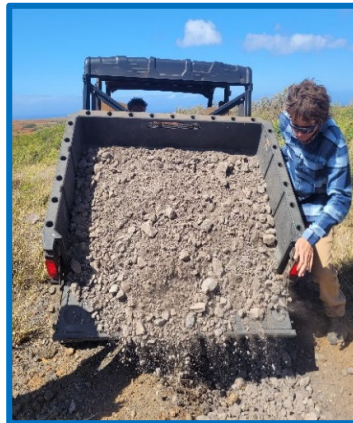
Top Left: Bert Lum and crew doing road work. Top Right: Seed collection at Wailuna. Top Middle: Gravel being dropped for road repair.
