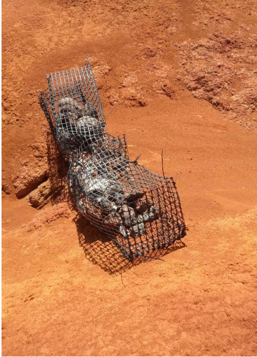
Gabion capturing sediment after a rain event
